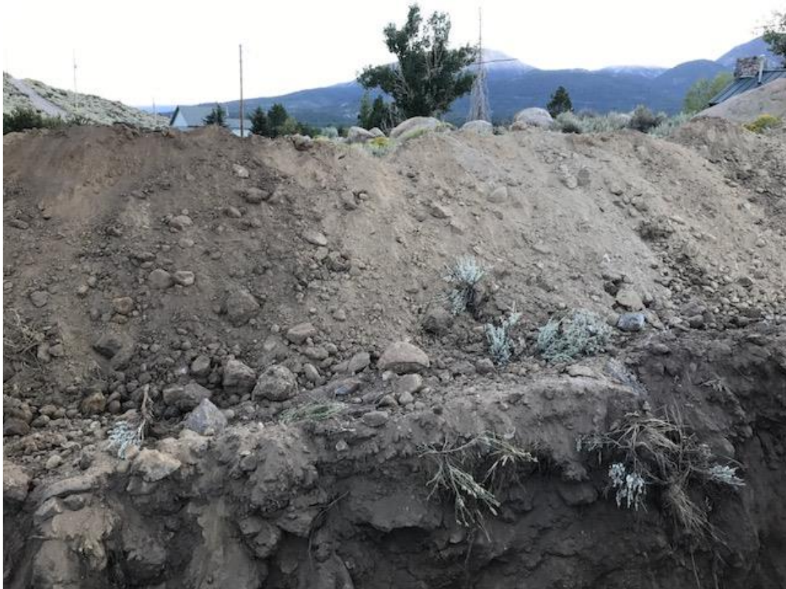
Photo 1 – South wall of trench along west side of Ascenté property boundary, showing fault trace, as seen by change in sediment color. NOTE were not scraped smooth, as is good professional practice.
